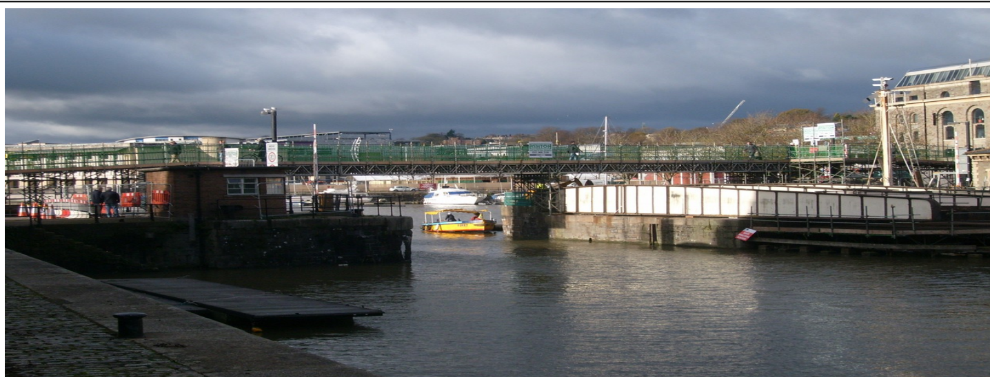
The Prince Street Bridge currently under repair with temporary scaffolding bridge above.
